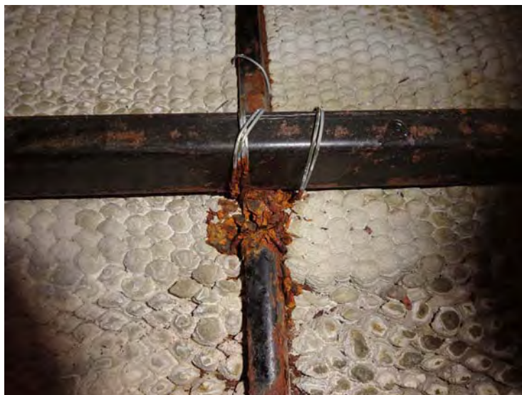
Examples of damage to metal supporting soffit stucco
