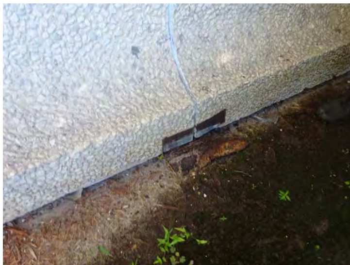
Examples of rusted and missing steel wall connecting plates. Also note gaps under wall where bugs and insects can enter.
