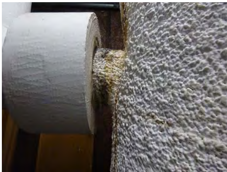
Examples of condensation leaking from chilled water piping insulation
