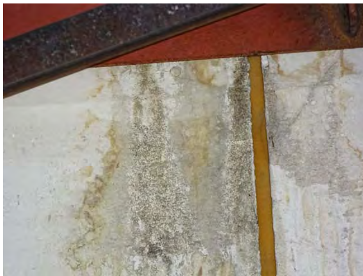
Examples of water stains on interior sides of fascia panels
