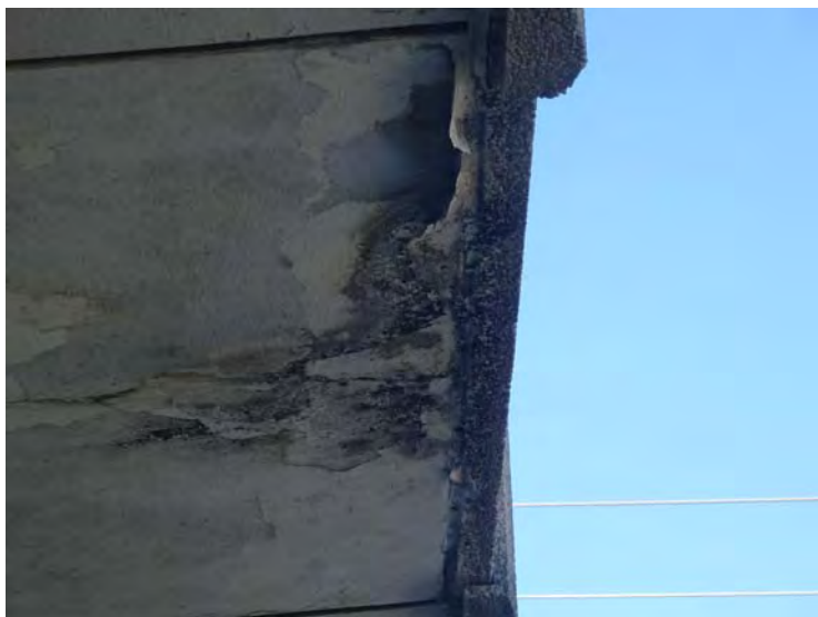
Examples of damage at underside of soffit
