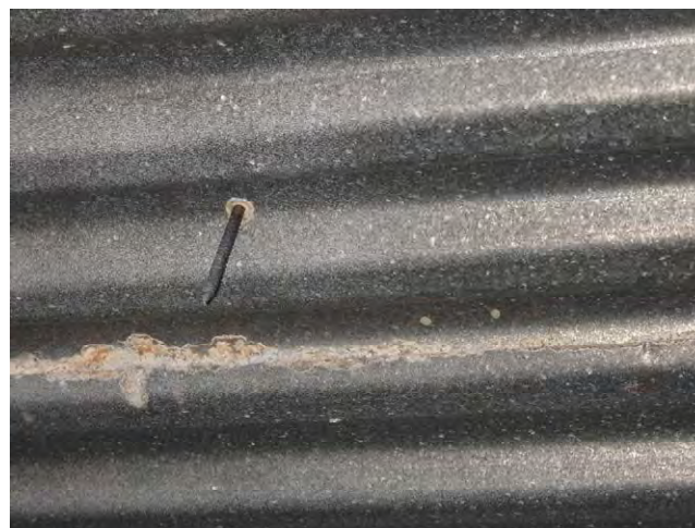
Picture 5 – Corrosion of Deck at Fastener Penetration
