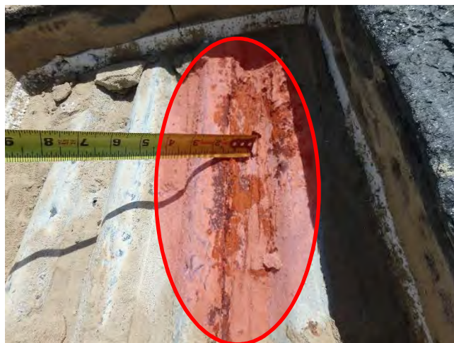
Picture 8 – Corrosion of Metal Deck
