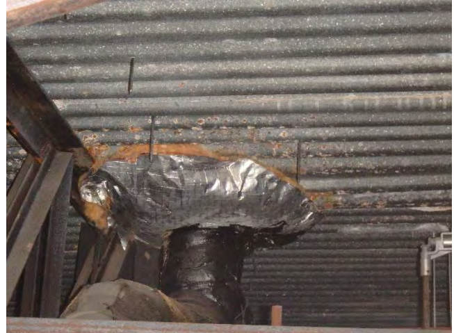
Picture 2 – Damaged Roofing Around Drain
