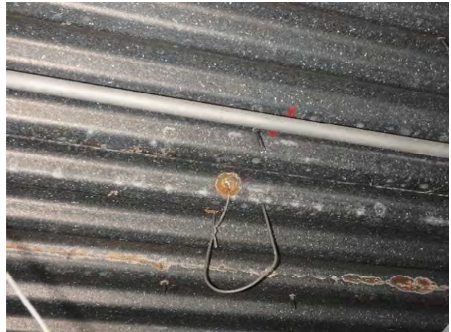
Picture 4 – Corrosion at Penetration
