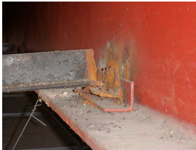
Picture 12 – Example of Detached Bracing
