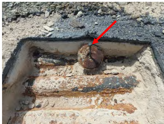
Picture 9 – Corrosion at Penetration
