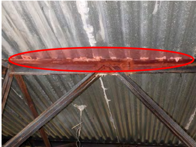
Picture 3 – Minor Corrosion of Main Truss
