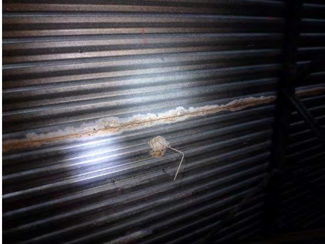
Picture 1 – Deck Damage at Panel Seam
