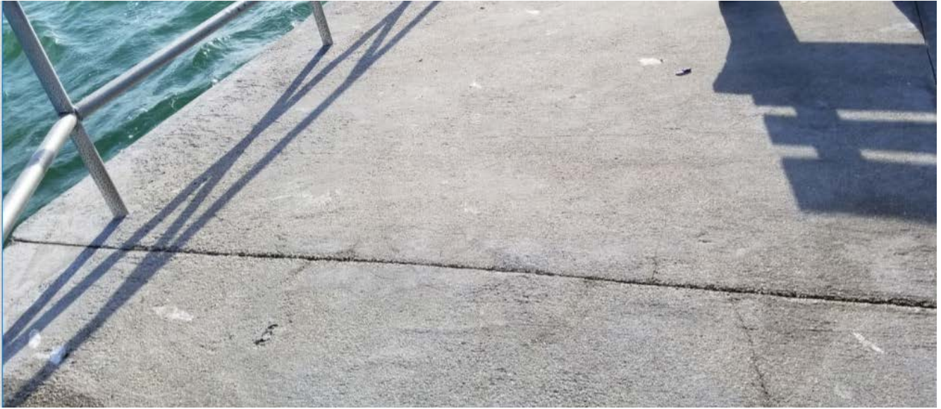
Figure 2-3 Typical Deck Condition
