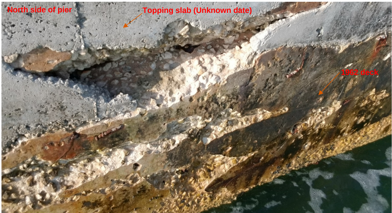
Figure 2-7 Deck Perimeter Spalling
