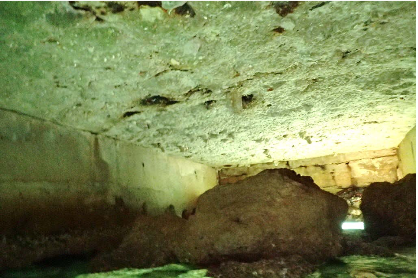
Figure 2-4 Typical Deck Underside Condition
