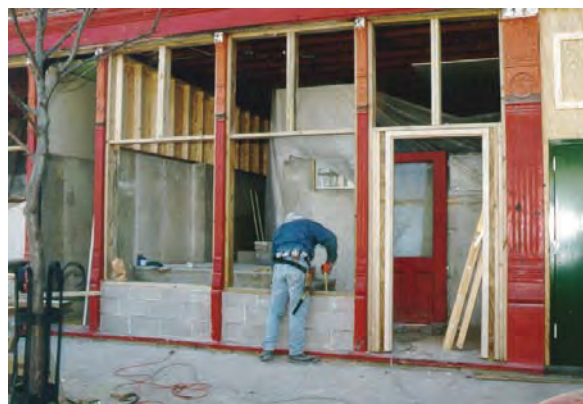
Floodproofing the vestibule of a storefront
