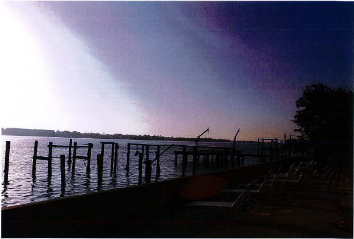
Figure 4. Storm Damaged Dock at 1605 Pass-A-Grille Way
