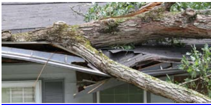
Hazardous fallen tree
