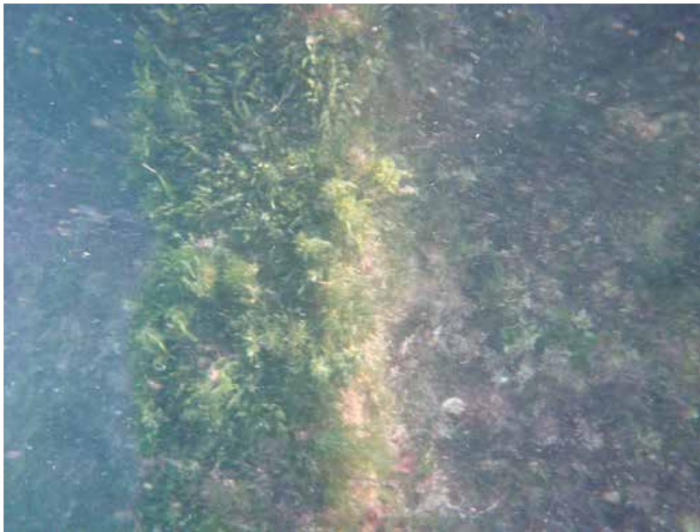
Representative algal cover on pier structure supports.
