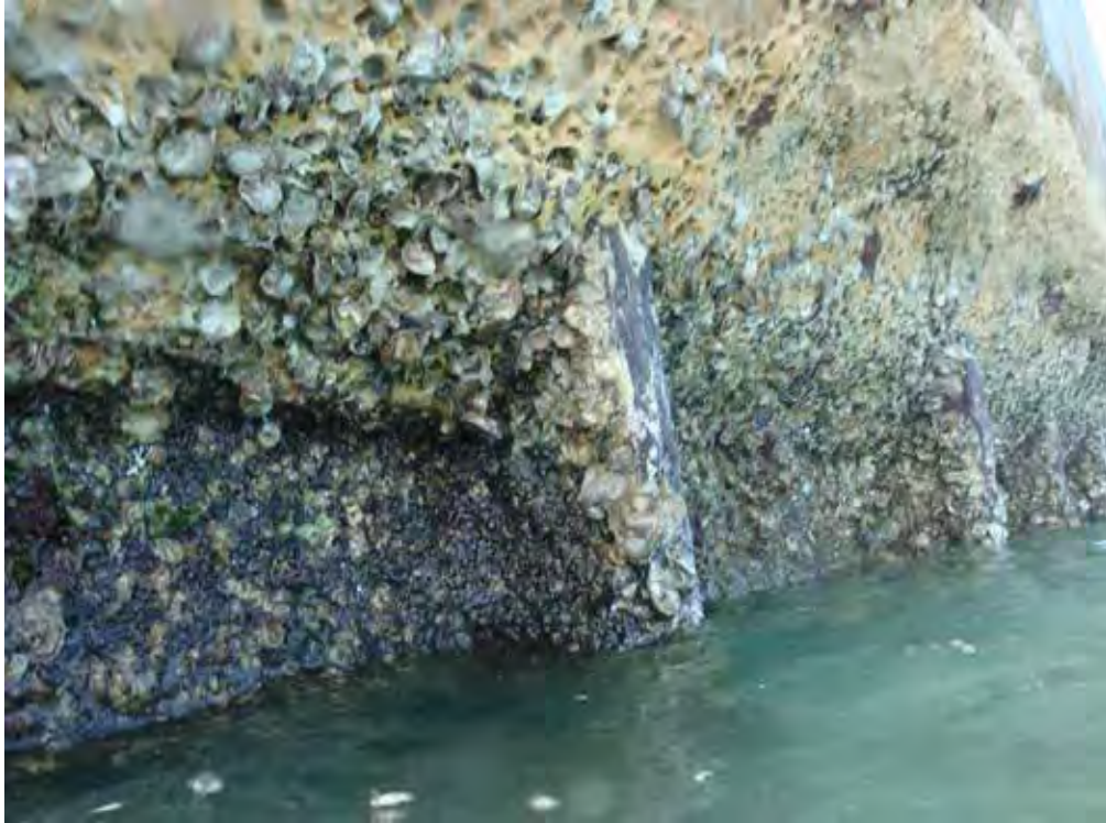
Typical fouling community on the structure at the water line.
