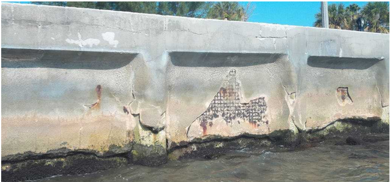
Figure 3-6 Loss of Shotcrete Exposing Mesh
