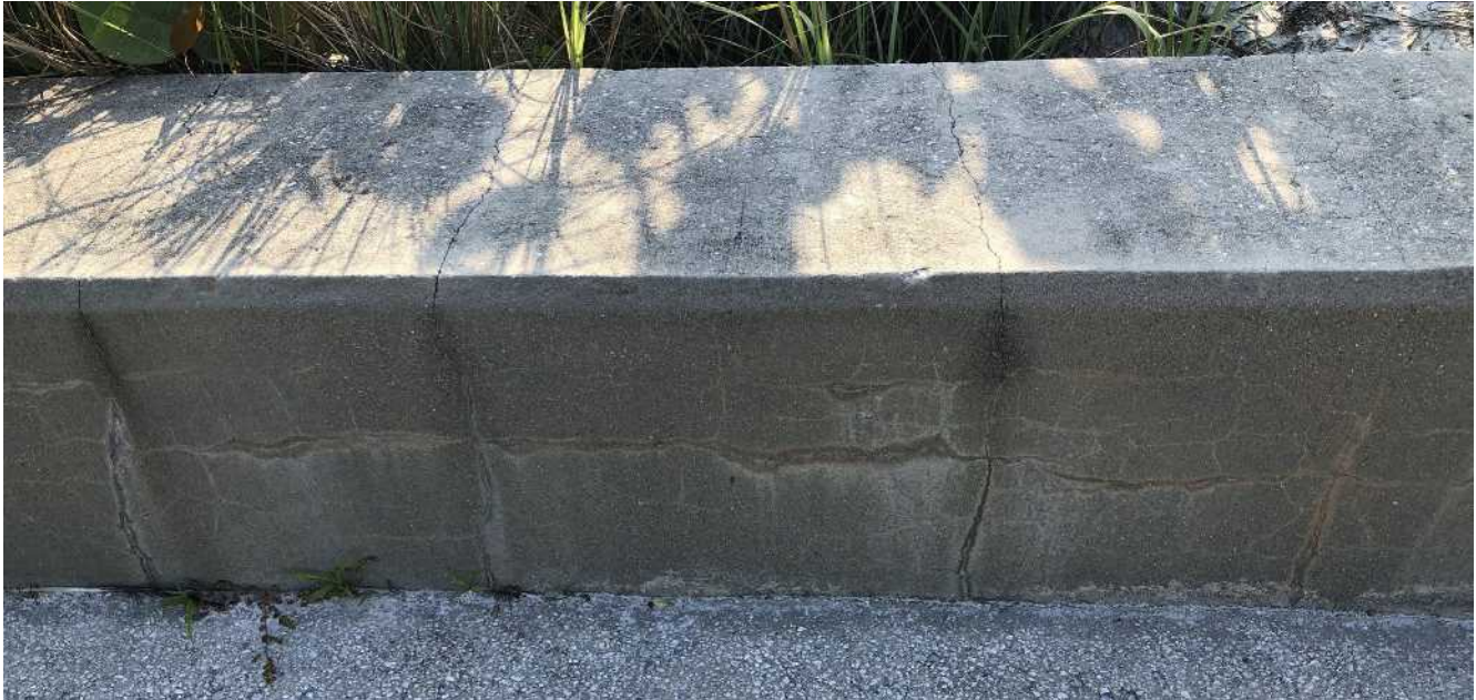
Figure 3-1 Typical Transverse Cracks, Station 1+00
