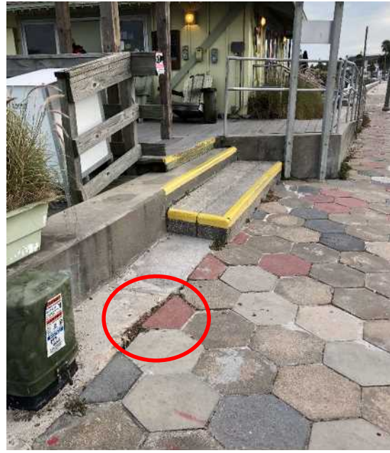
Figure 7: Void under the Sidewalk
