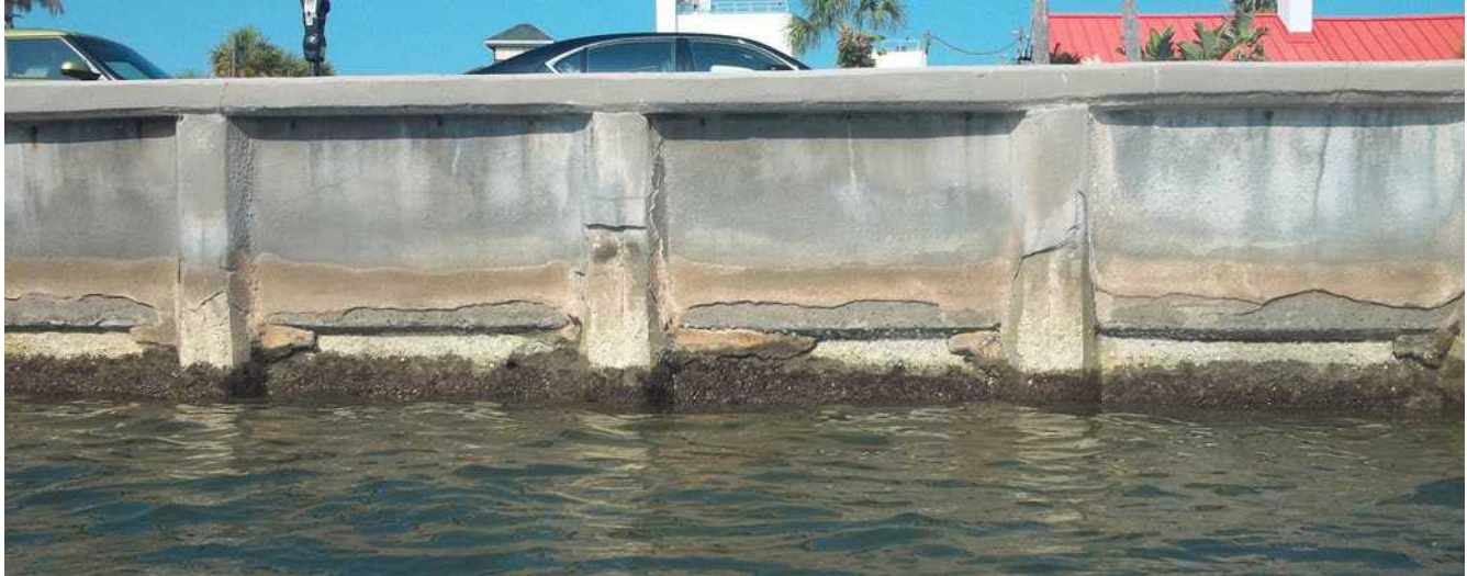
Figure 3-5 Loss of Shotcrete
