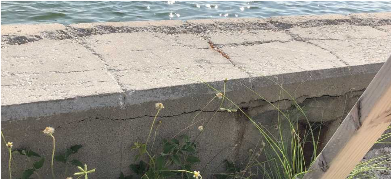
Figure 3-3 Longitudinal cracks in Cap with Corrosion Bleedout
