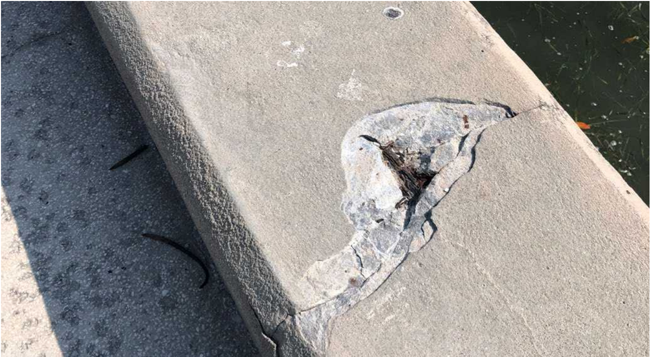
Figure 3-7 Spall with Exposed Rebar
