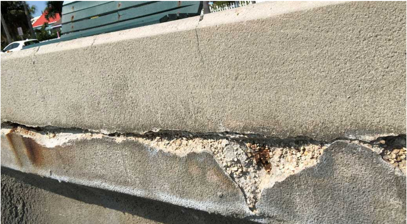
Figure 3-4 Longitudinal Cracks with Spalling
