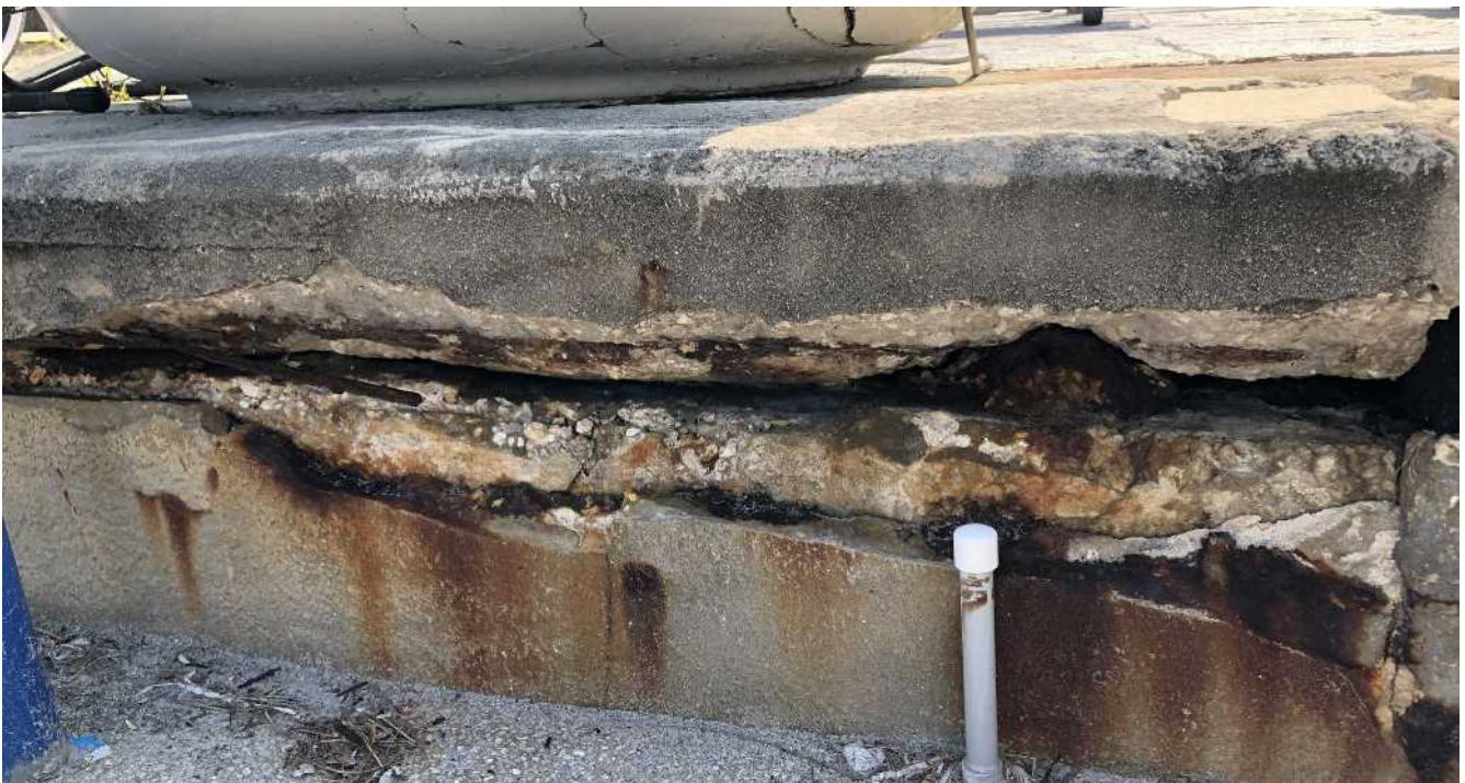
Figure 3-8 Severe Spall, Exposed Rebar with Complete Section Loss
