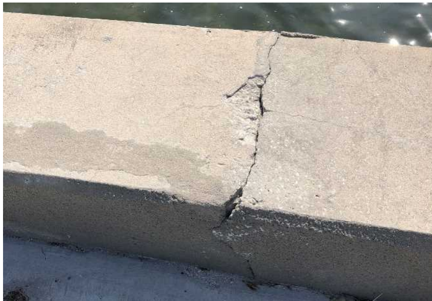
Figure 3-2 Severe Transverse Crack, Station 15+00
