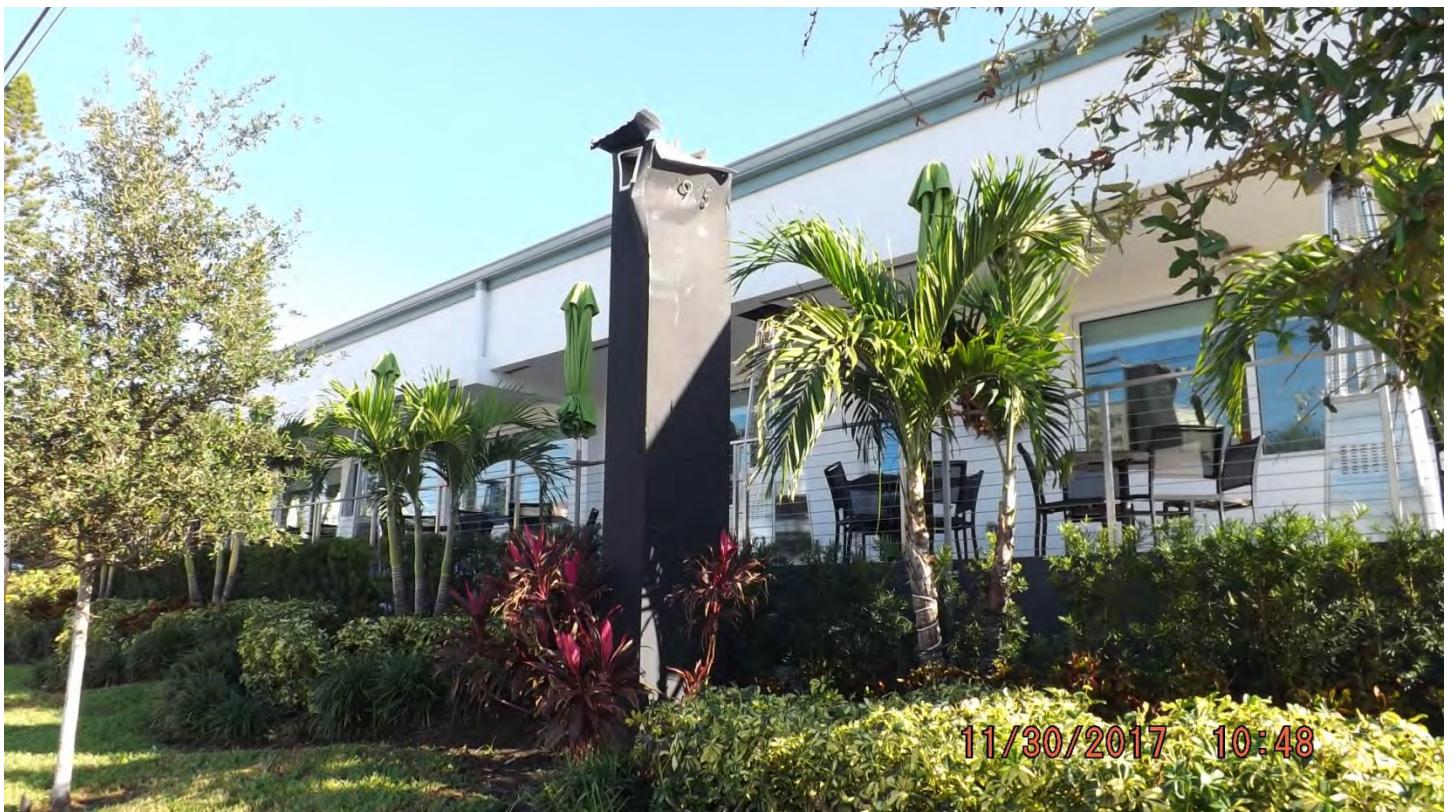
Above: Subject property, facing northeast. Damaged sign structure in center.
