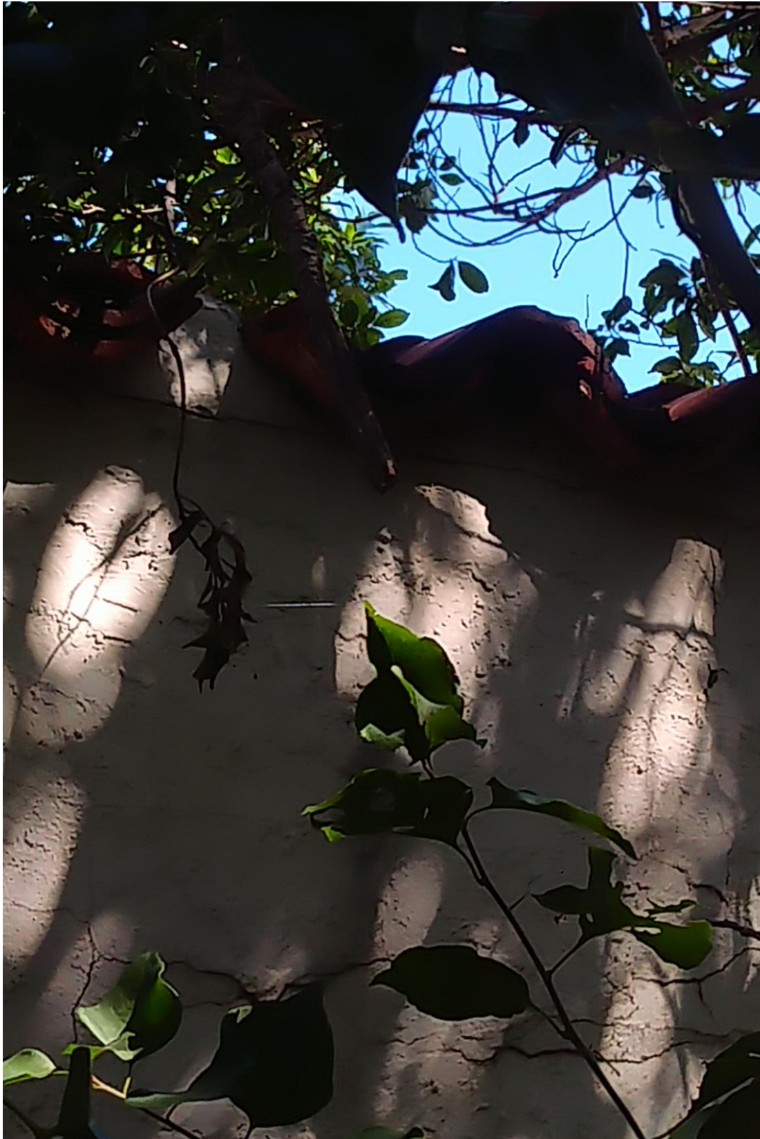
Continuous Perimeter Cracking Below Roof Tiles
