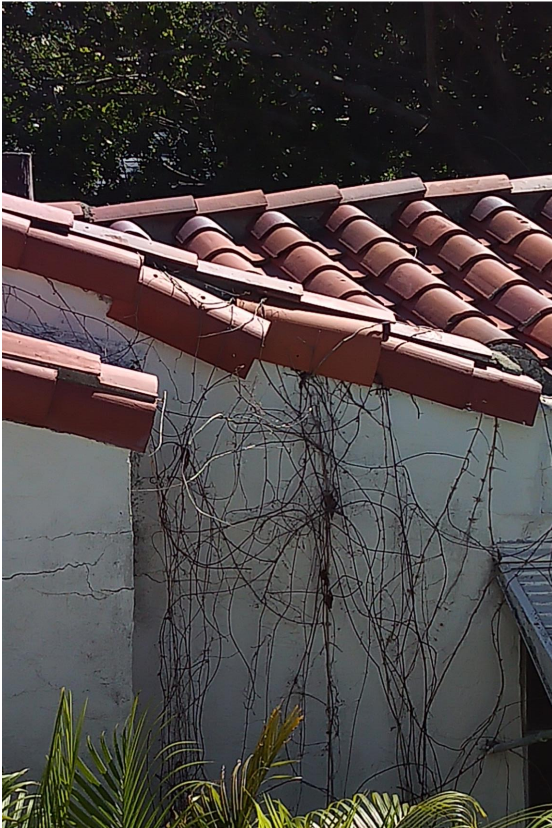
Failing Ridgeline of Roof
