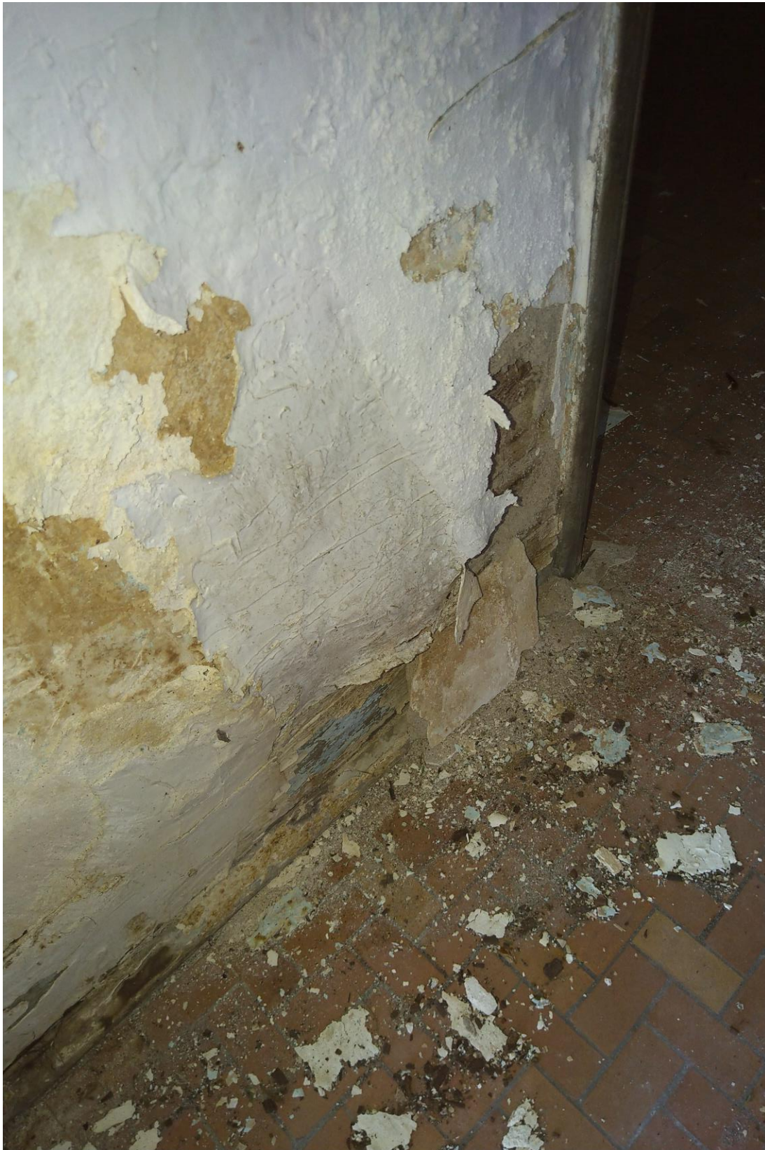
Interior Walls Damage
