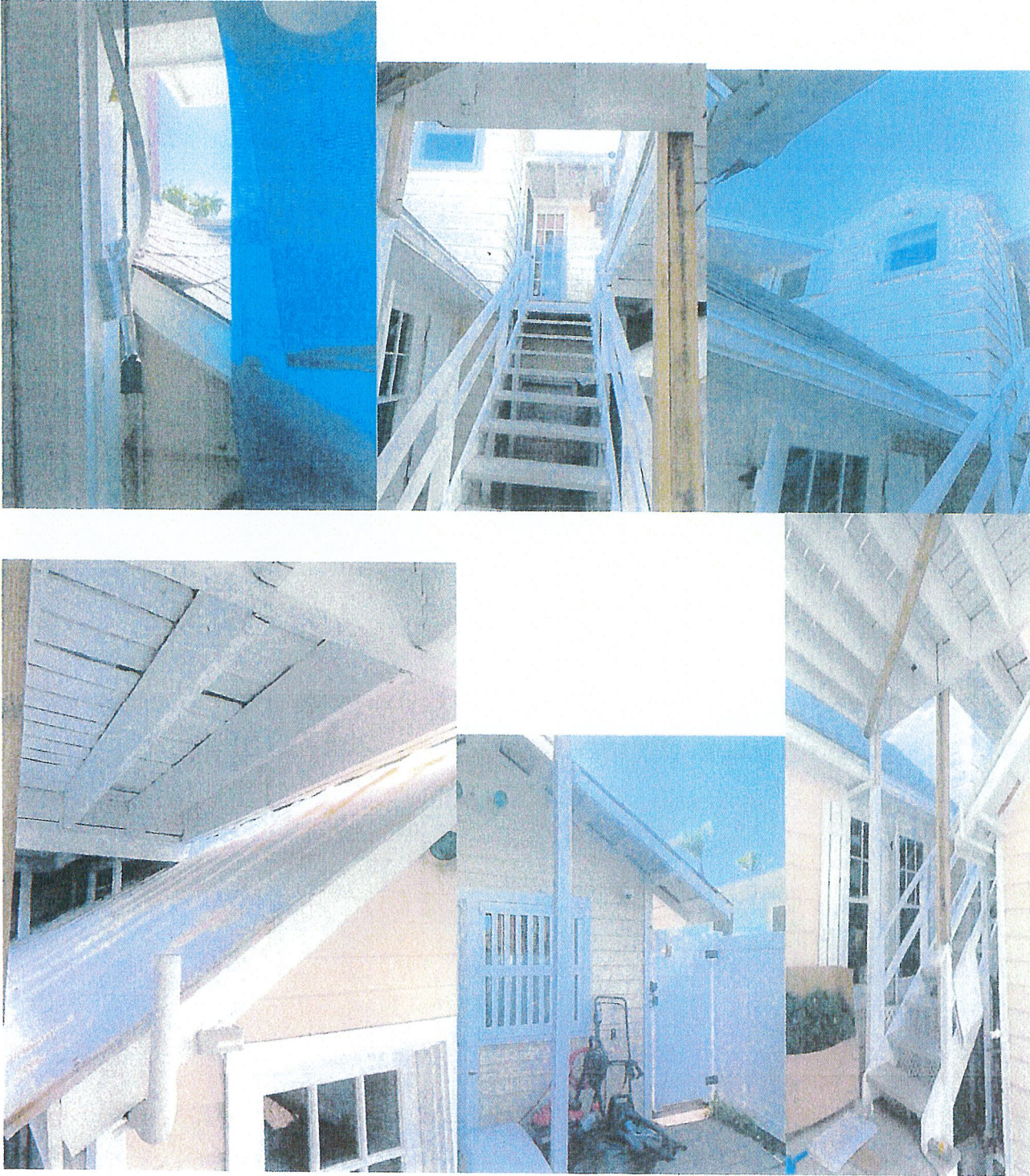
VARIOUS REAR BUILDING VIEWS W/ MANY ALTERATIONS
