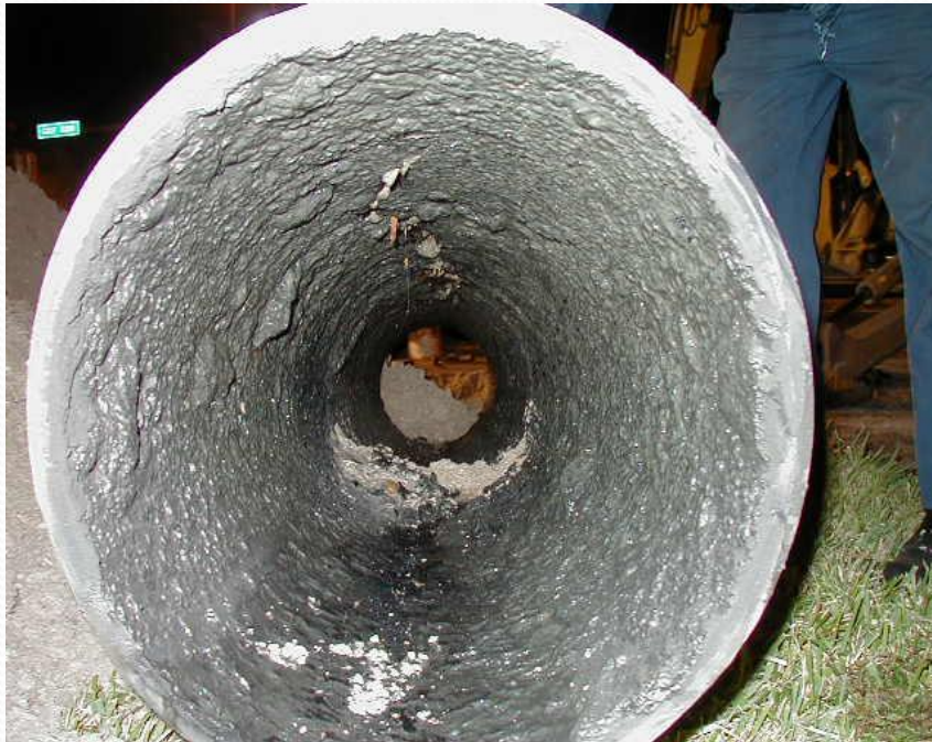
Major Pipe Failure
