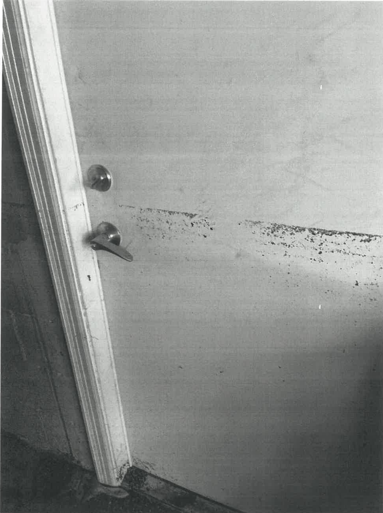
Waterline 39" the living space is destroyed and outside dock, fences, decks, masonry walls
