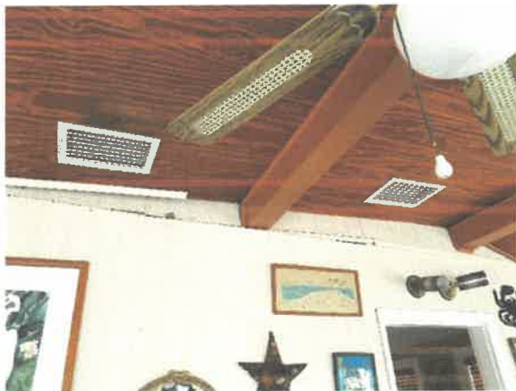
Observation 7: Cracking at top of wall joint line
