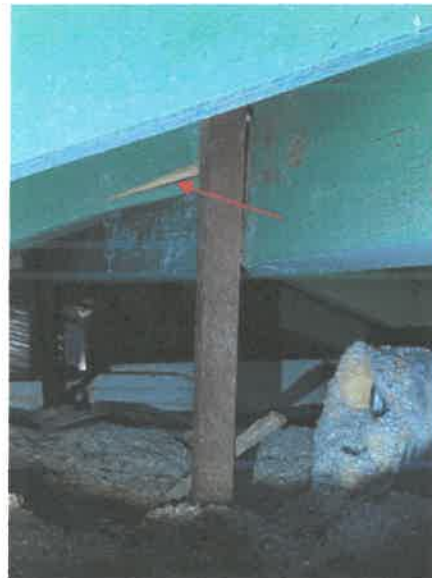
Observation 4: Cracking on rafter
