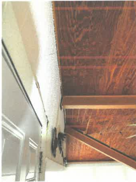
Observation 9: Bowing wall at front entry
