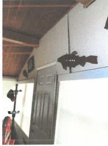
Observation 10: Bowing wall at front entry
