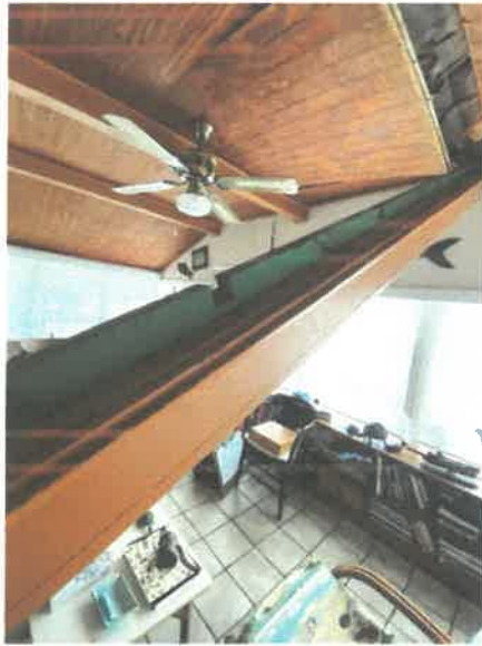
Observation 1: Fallen beam at front entry
