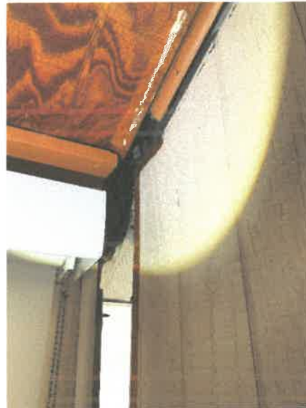
Observation 8: wall corner separation
