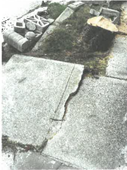
Observation 13: Cracked slab Non-Structural
