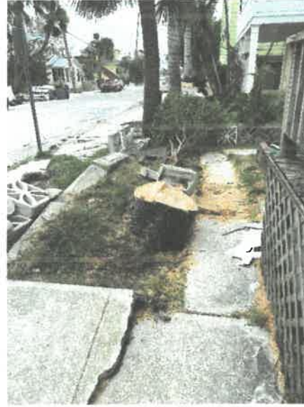
Observation 14: Cracked slab
