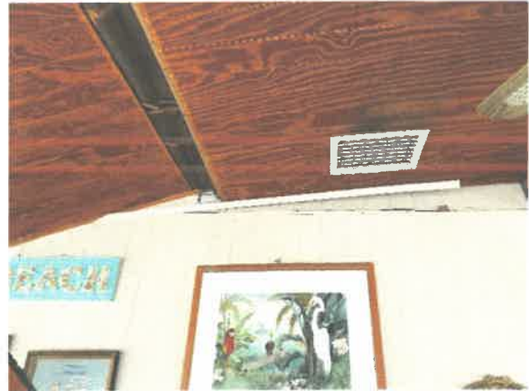
Observation 6: Cracking at top of wall joint line
