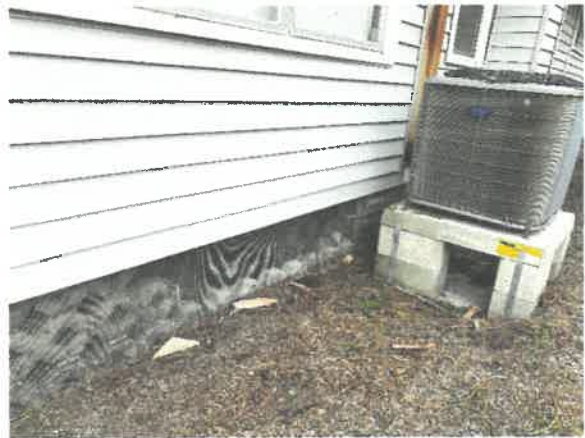
Observation 12: Fallen concrete blocks Non-structural
