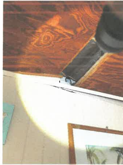
Observation 2: Connection beam to wall
