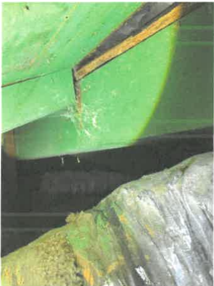
Observation 3: Rafter to Ridge beam failed connection
