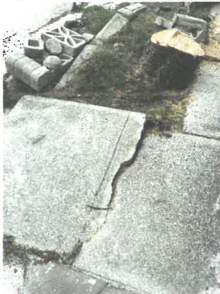
Observation 13: Cracked slab Non-Structural
