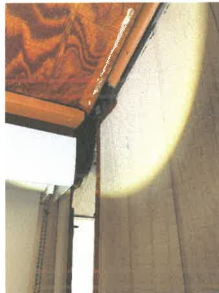
Observation 8: wall corner separation
