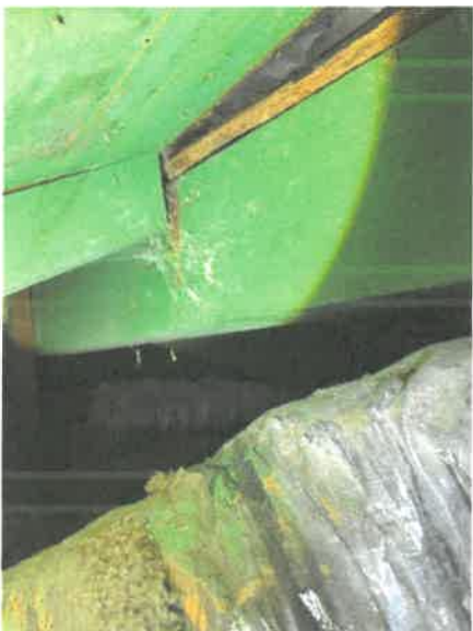
Observation 3: Rafter to Ridge beam failed connection
