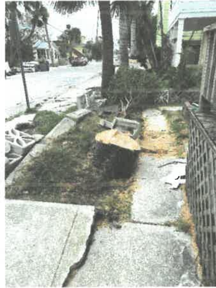
Observation 14: Cracked slab
