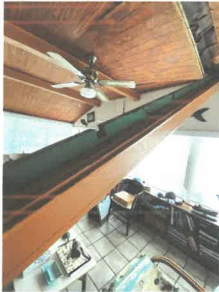
Observation 1: Fallen beam at front entry
