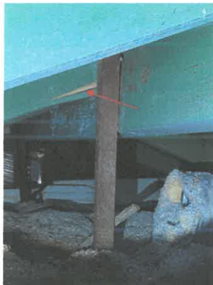
Observation 4: Cracking on rafter
