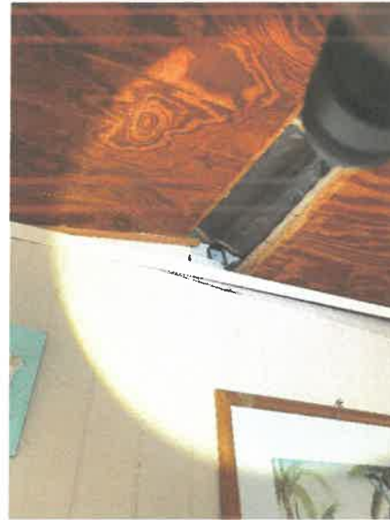
Observation 2: Connection beam to wall
