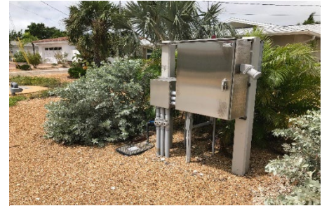
Figure 20: St. Pete Beach Lift Station
