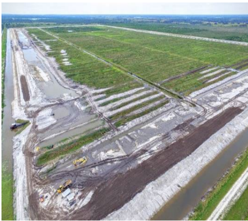
Figure 11: Aerial View of the SFWMD C-23 Section C Water Farm AGI
