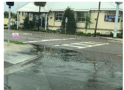
Figure 21: Tidal Flooding at Boca Ciega Drive in St. Pete Beach
