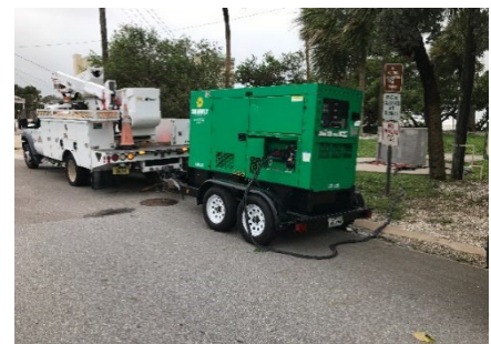
Figure 16: St. Pete Beach Backup Generator
