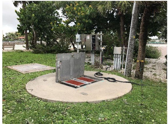
Figure 13: St. Pete Beach Sanitary Sewer Lift Station #10
