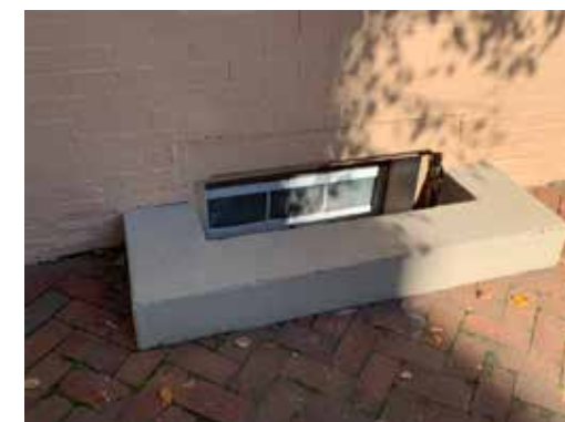
[55] A low flood wall or curb that is compatible with the historic character of the property can be constructed around basement windows to keep flood waters out. Photo: Jennifer Parker/NPS
