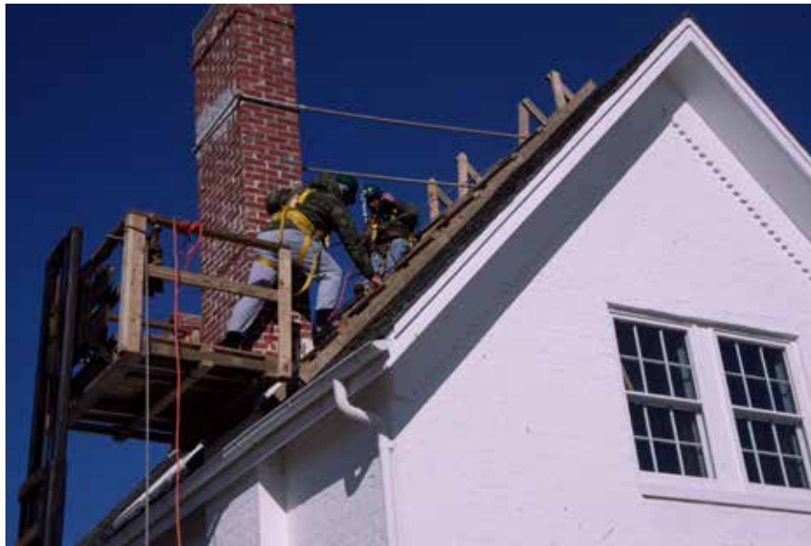
[113] Fragile features like chimneys should be evaluated and braced before a building is moved. Photo: Mike Booher/NPS
