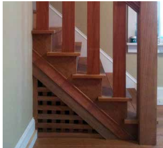
Figure 3: Instead of solid wall material, an open lattice was installed under the stair to vent an otherwise inaccessible space. Photo: Mary Delaney Krugman, JD, MSHP
