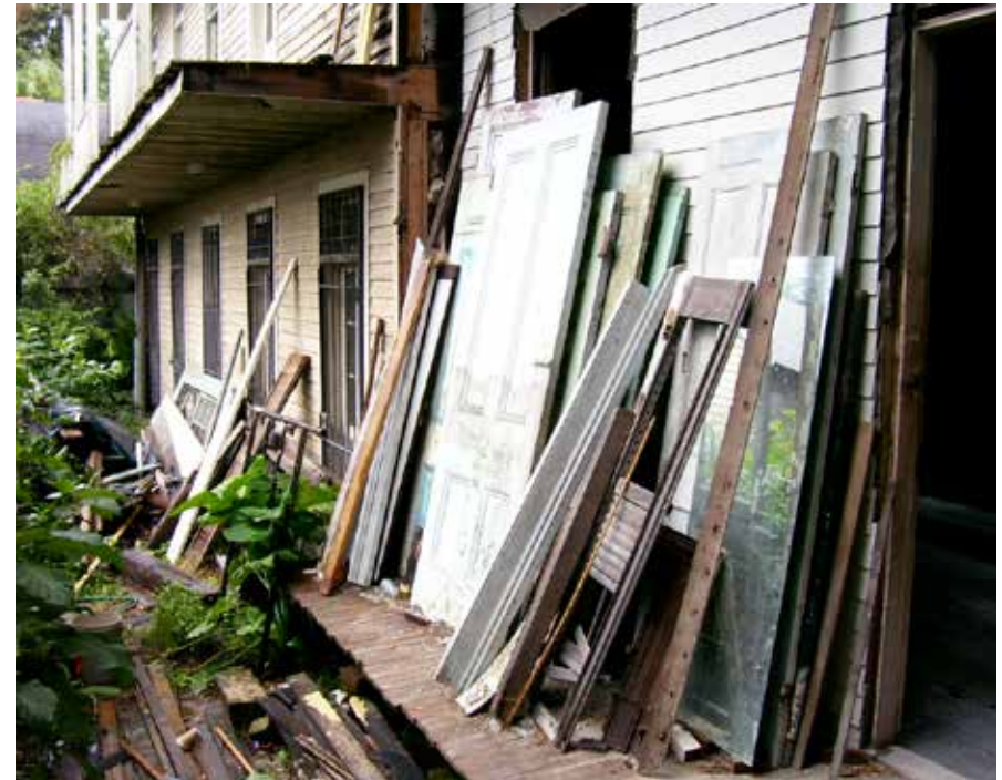
[120] If a property is demolished, carefully salvaging historic materials can help other historic properties undergoing rehabilitation and give a 'second life' to these otherwise lost materials. Photo: Jenifer Eggleston/NPS
