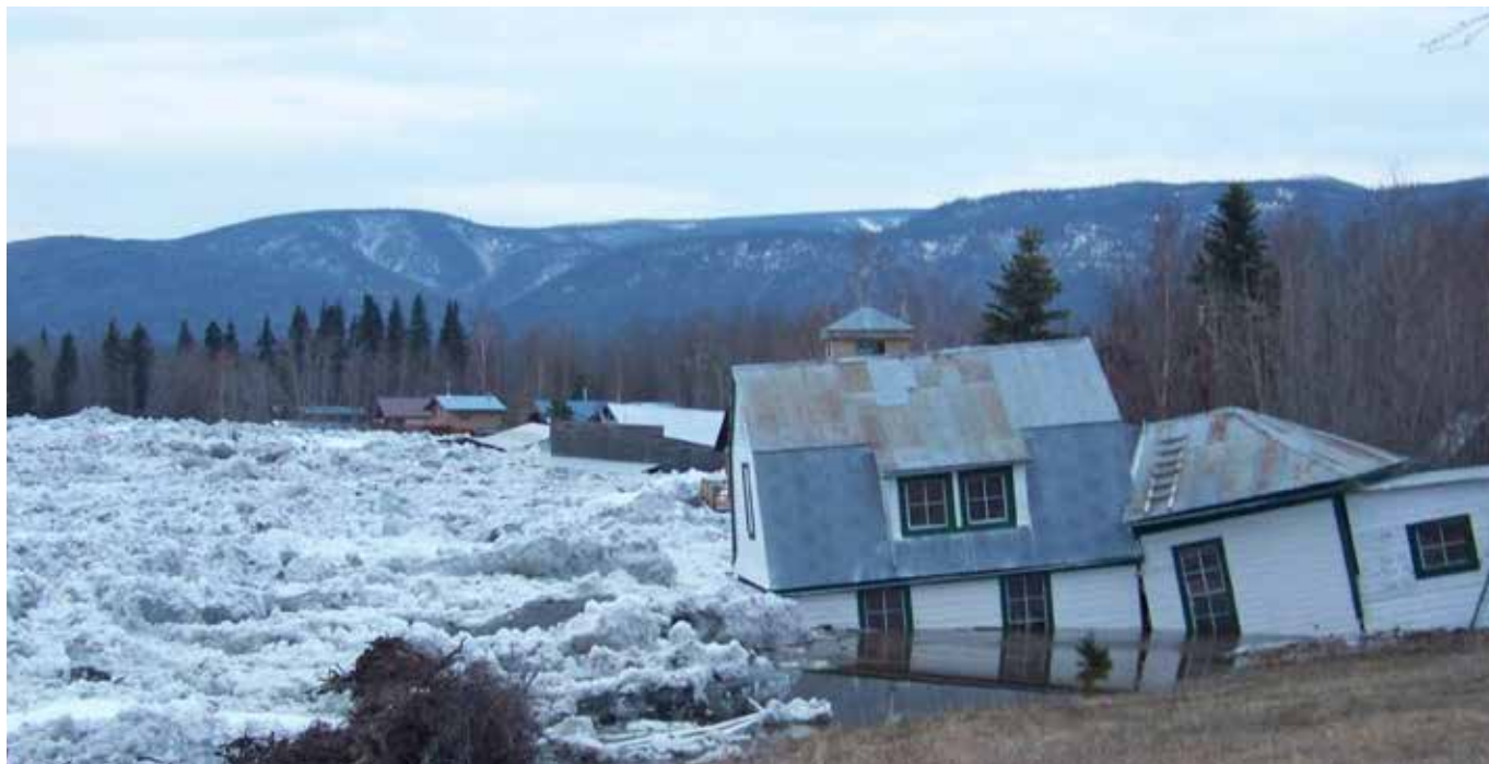
[5] In 2007 the Old Customs House located in the Yukon-Charley Rivers National Preserve, AK, was significantly damaged by riverine flooding. Historic properties that may not have flooded before are increasingly affected by larger flood events. Photo: Carl Stapler/NPS
