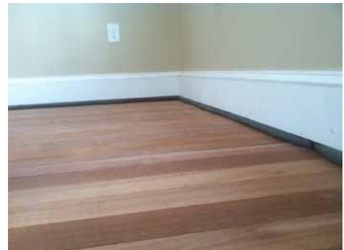
Figure 5: Mahogany wood floor and baseboard with a gap at the base for future venting. Foam insulation strip fills the gap and will be covered with removable trim. Photo: Mary Delaney Krugman, JD, MSHP
