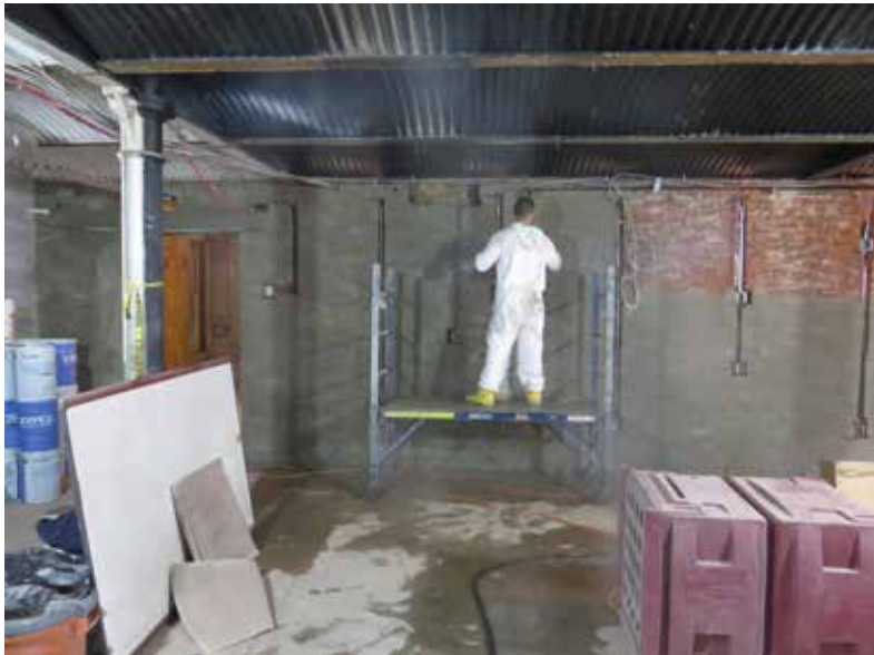
[48] A waterproof coating is applied to the interior surface of lower-level walls of the public library in Hoboken, NJ. Prior to applying such a coating, the product should be researched by building science professionals with knowledge of historic materials and methods to ensure that the coating will not cause damage to or accelerate deterioration of the structure. Photo: David V. Abramson for Hoboken Public Library
