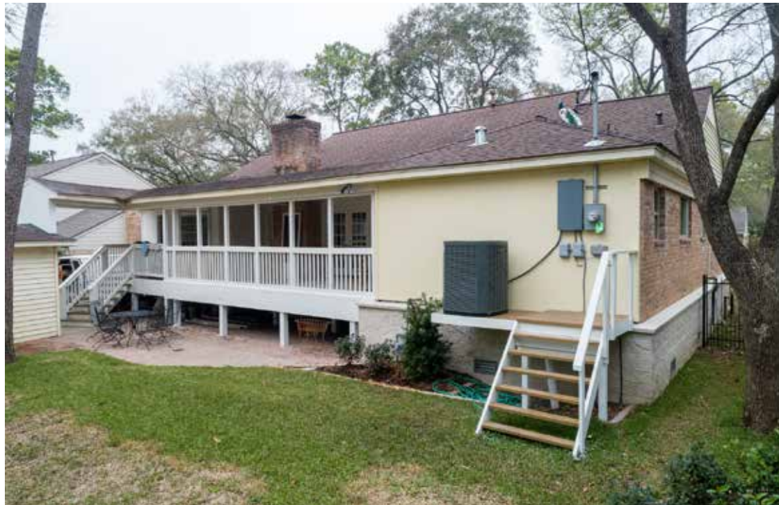
[44] Access issues must be considered when relocating exterior mechanical equipment on an elevated platform. If electrical or gas meters are moved to higher locations, stairs or a ladder may be required by the utility company to facilitate meter reading. Photo: p3elevation.com
