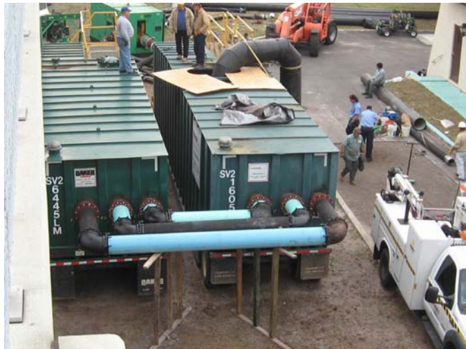
Settling Tanks at PS 61
