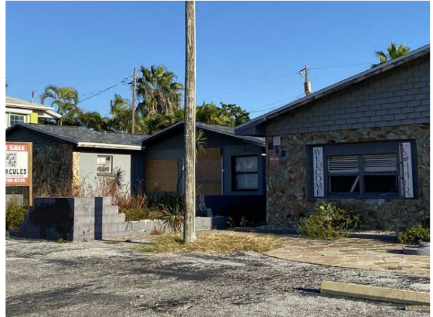
Figure 27 Vacant Residences, Severely Damaged, 73 rd Avenue.
