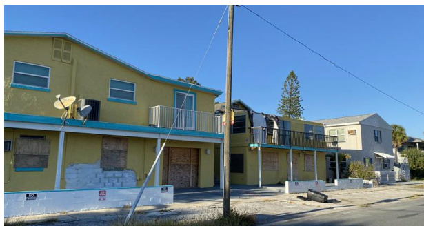
Figure 24 Severely Damaged Residential, 73 rd Avenue and Sunset Avenue.
