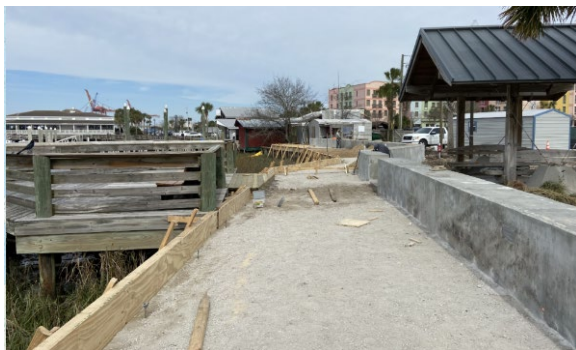
Figure 6 Boardwalk and Seawall Repair (Amelia River Waterfront CRA)
