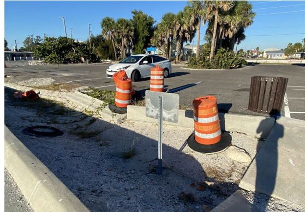
Figure 18 Sunset Park Seawall and Parking Lot Damage
