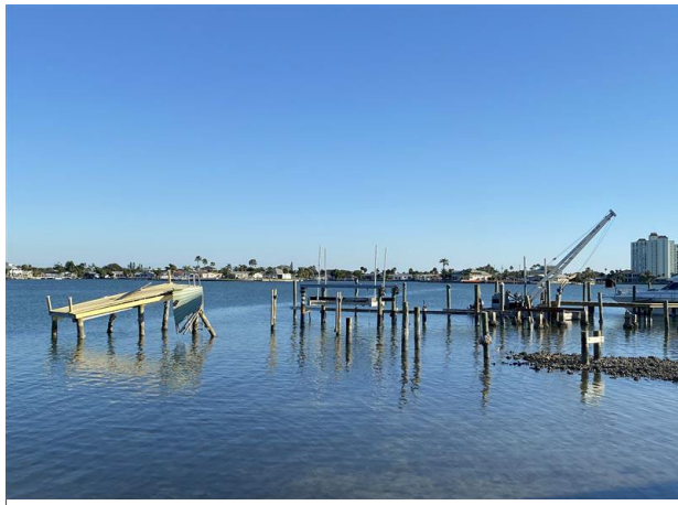
Figure 19 Bay St and Corey Avenue Dock Damage
