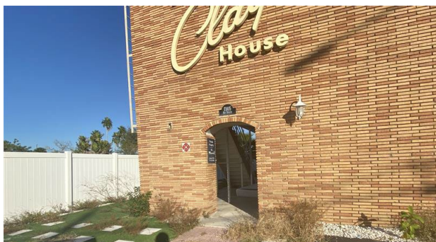
Figure 22 Clay House Residences, Severely Damaged, Bay Street and 73 rd Avenue.
