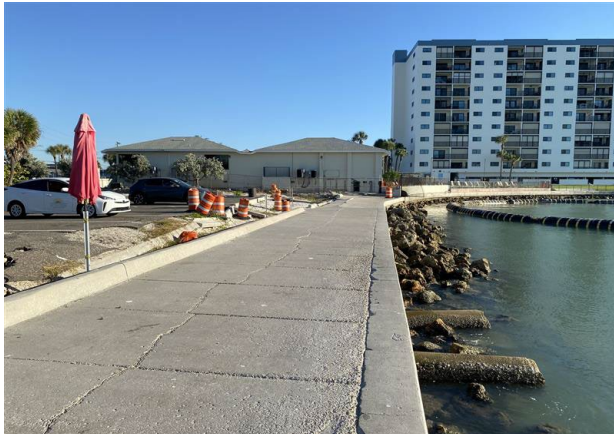
Figure 17 Sunset Park Seawall Damage
