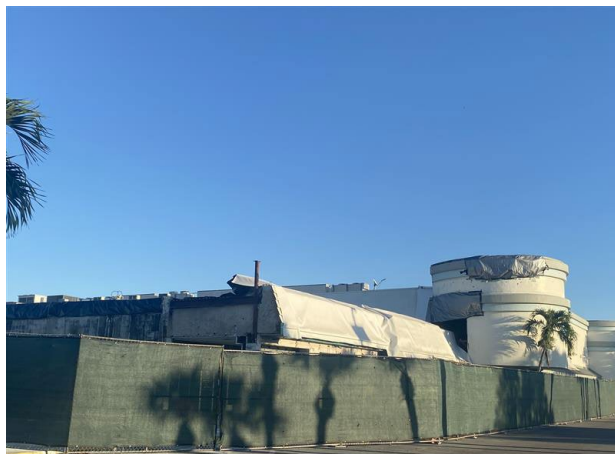
Figure 21 Publix Damage, Currently Closed
