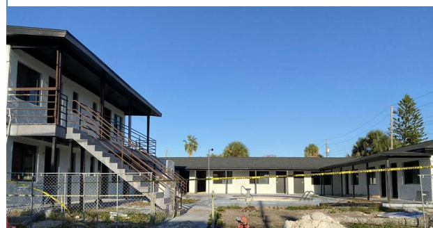
Figure 25 Severely Damaged Residential, Corey Avenue and Coquina Way.
