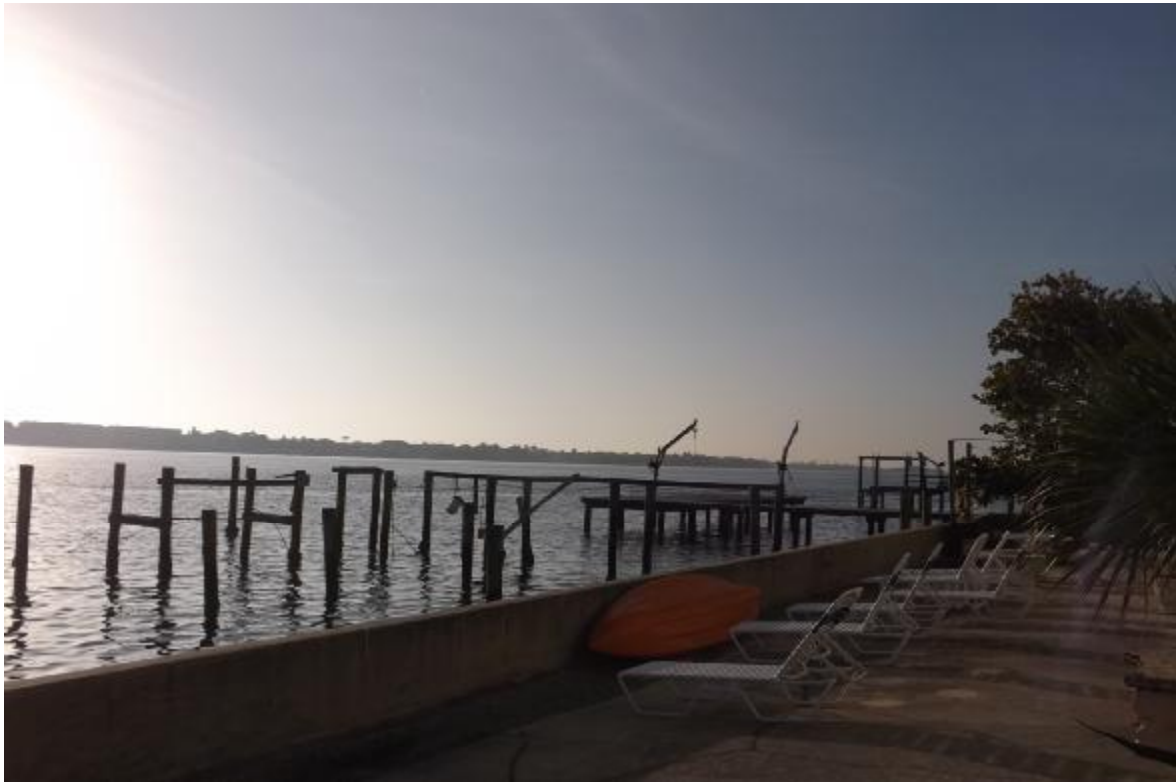
Figure 4. Storm Damaged Dock at 1605 Pass-A-Grille Way
