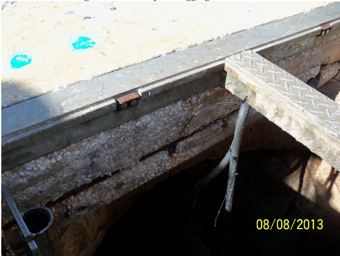
Figure 3 – LS#5 Exposed Aggregate and Rebar
