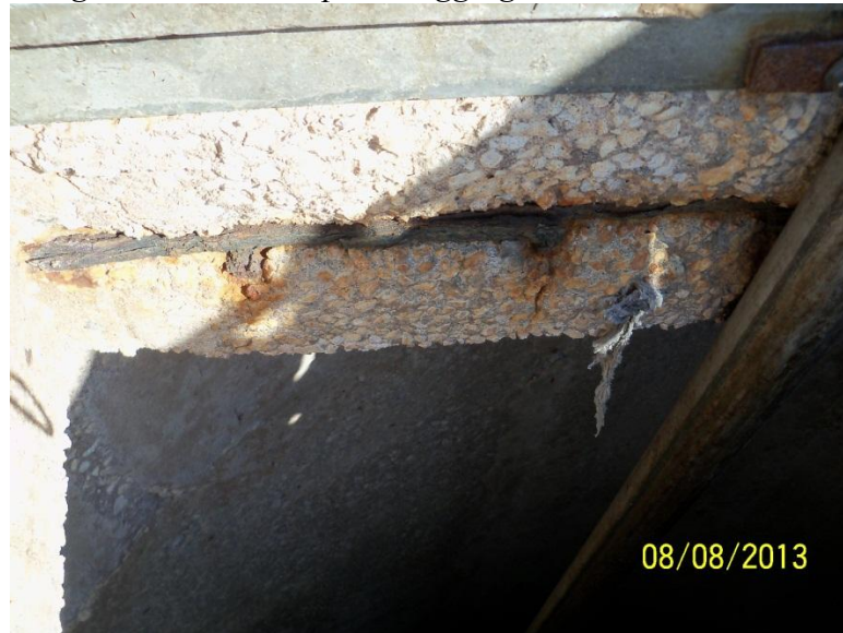
Figure 5 – LS #6 Exposed Aggregate and Rebar
