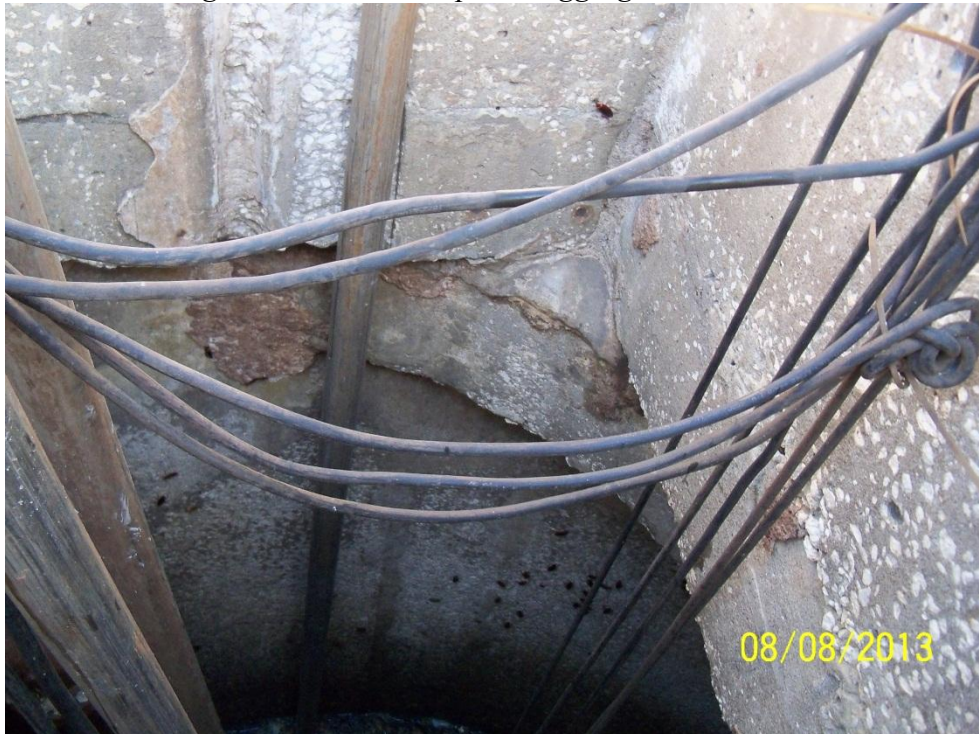
Figure 11 – LS#12 Exposed Aggregate and Rebar
