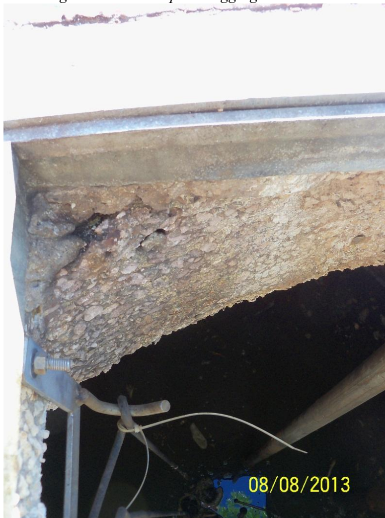
Figure 7 – LS#9 Exposed Aggregate and Rebar
